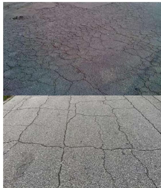
Fig1. Common problems in roads across all over the city.
